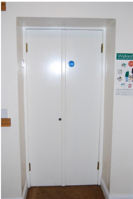
Figure 20: Internal fire door separating exhibition space from the rest of the building.
