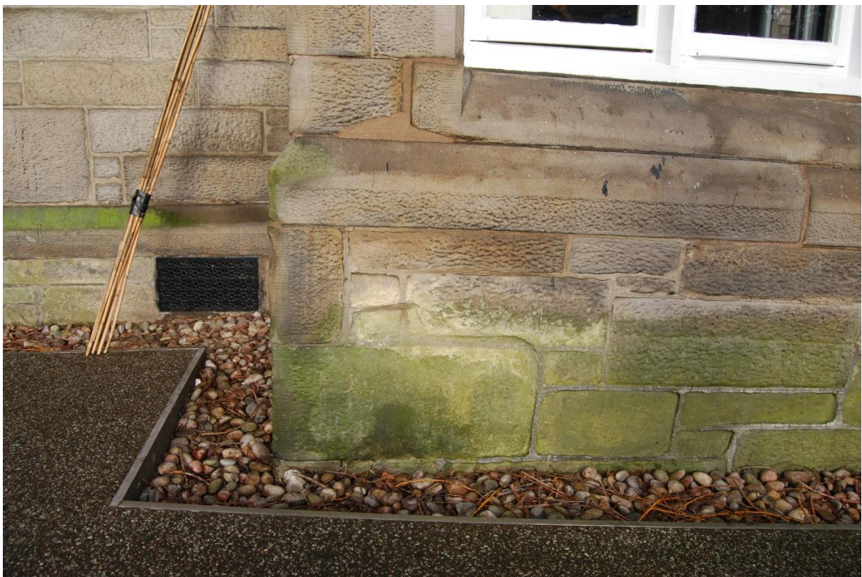
Figure 8: Greening of masonry caused by excess ground water.
