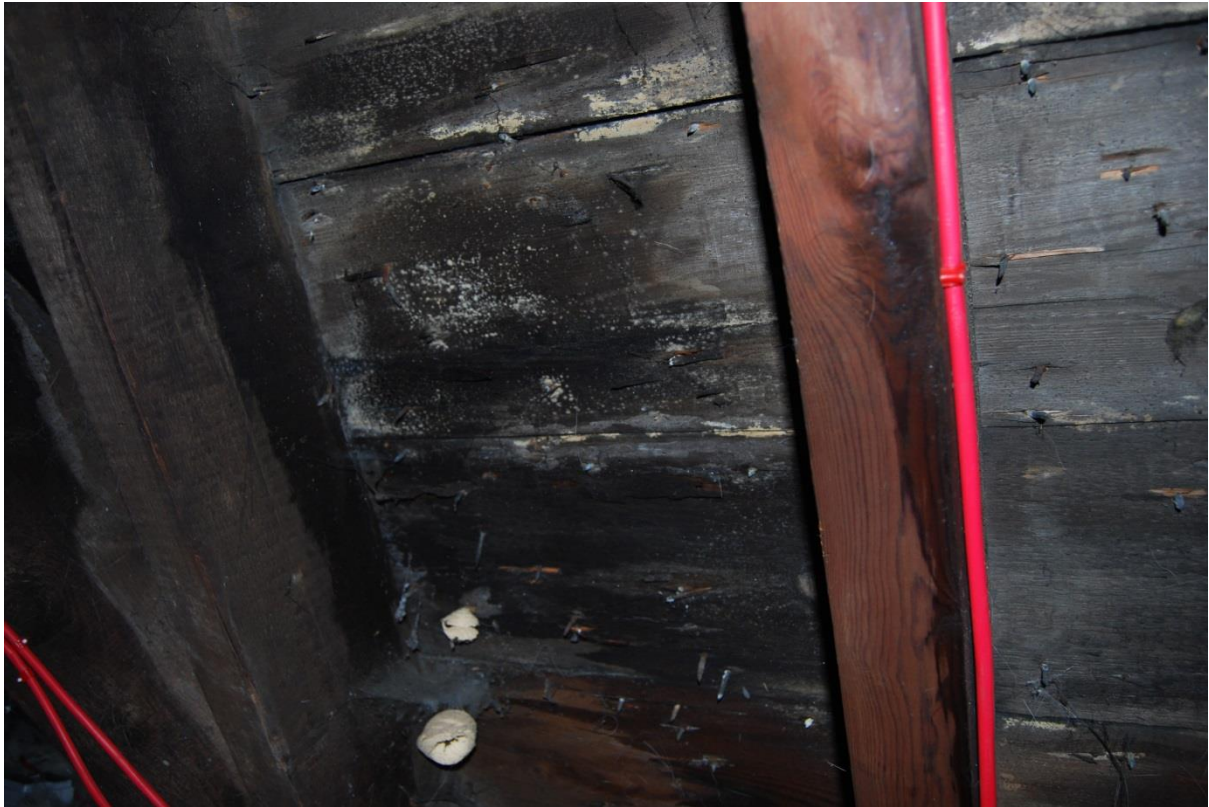
Figure 31: Underside of sarking in northern roof space showing signs of mould.
