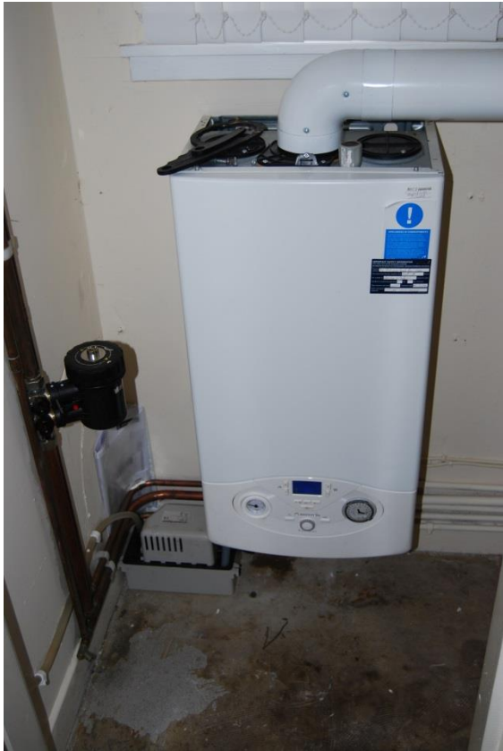
Figure 25: Existing gas boiler.
