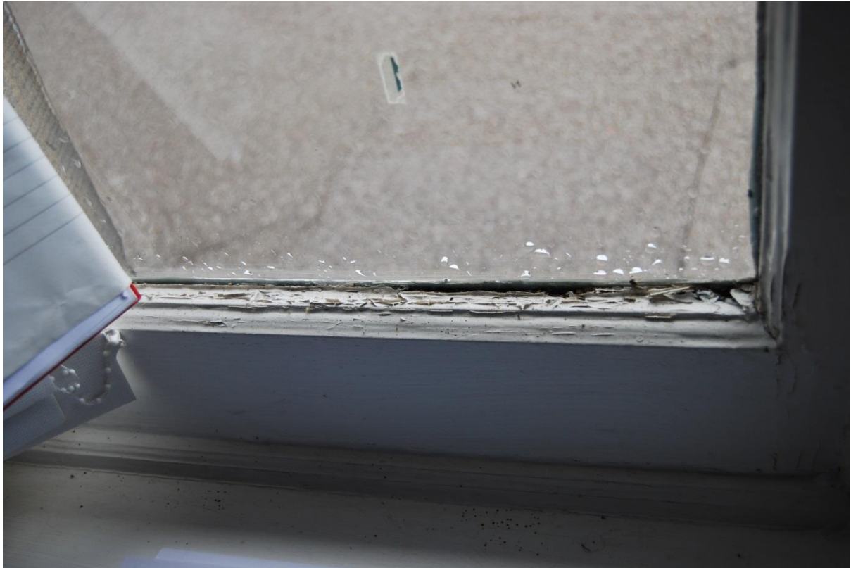
Figure 19: Early signs of rot on the interior of a window on the west elevation at ground floor level.
