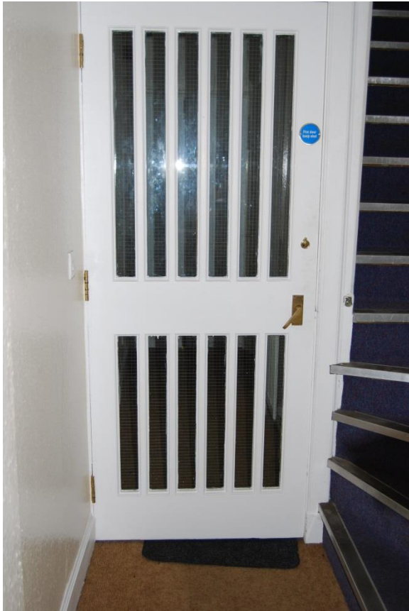
Figure 21: Internal glass and timber fire door separating the entrance hallway from the office space on the ground floor.
