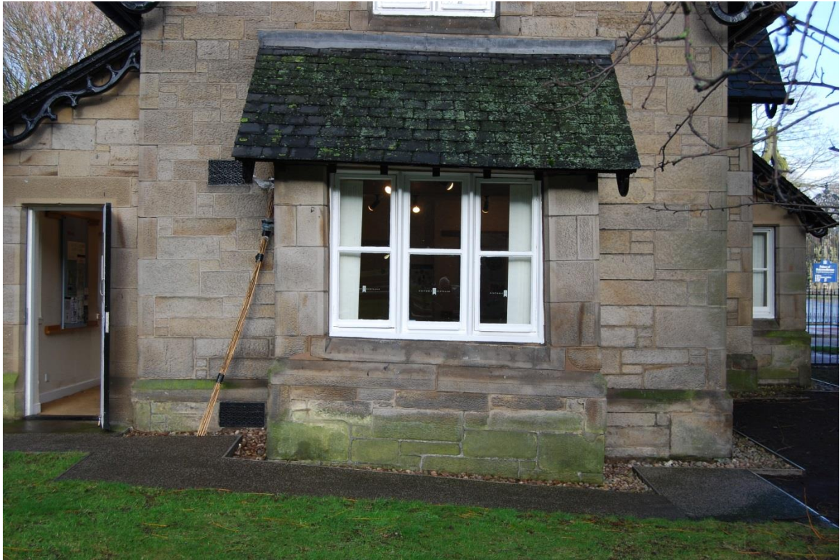
Figure 3: South elevation of the lodge showing signs of subsidence
