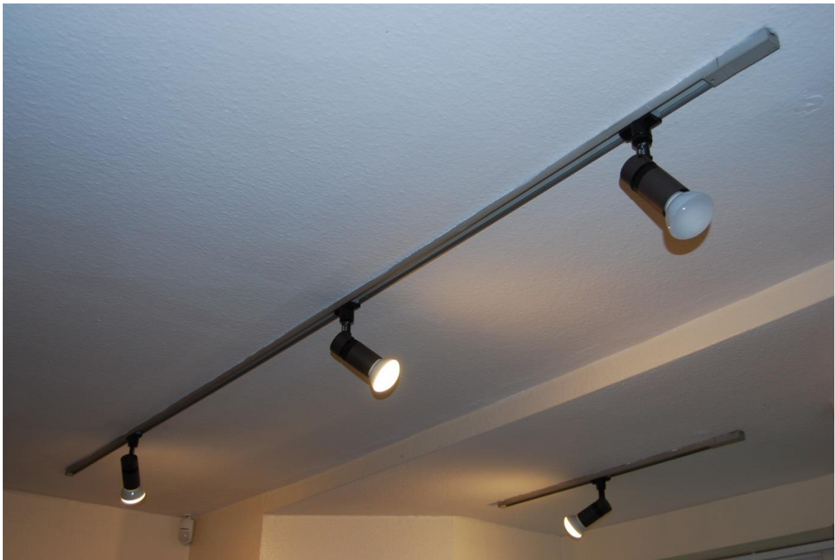
Figure 24: Existing spotlights in exhibition space and round floor office.
