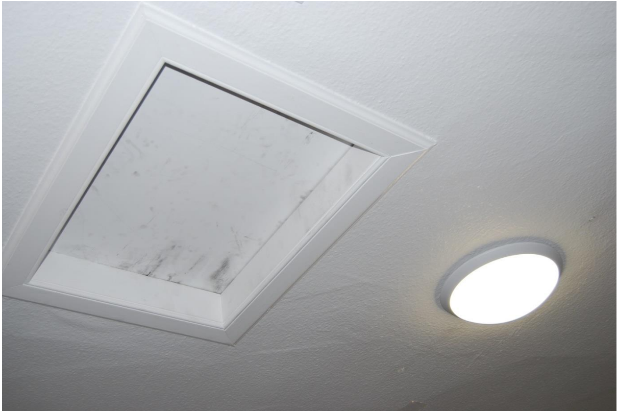
Figure 27: Slightly larger hatch in first floor storage room offering access to the southern attic space.
