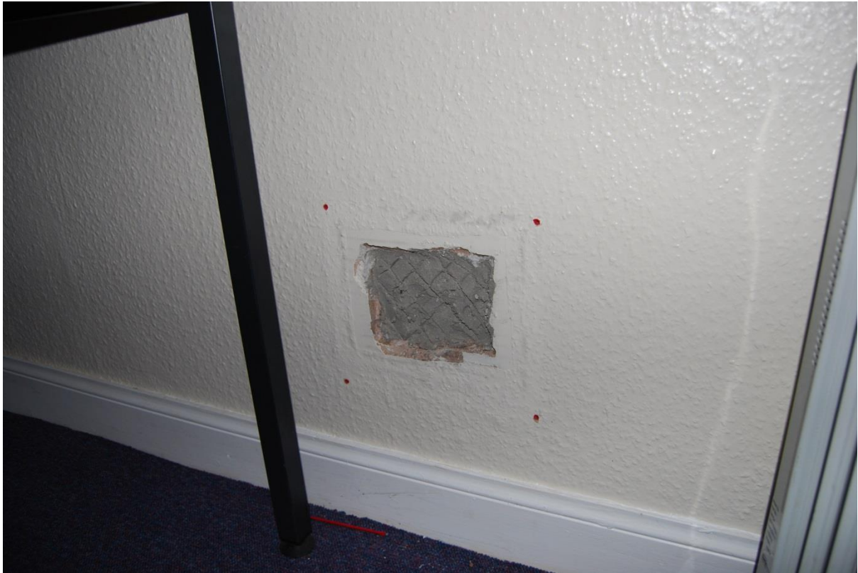
Figure 17: Blocked up vent in ground floor office, where original fireplace would have been.
