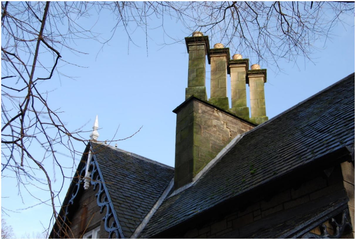
Figure 1: Diagonal crack in the masonry on the southern side of the chimney stack
