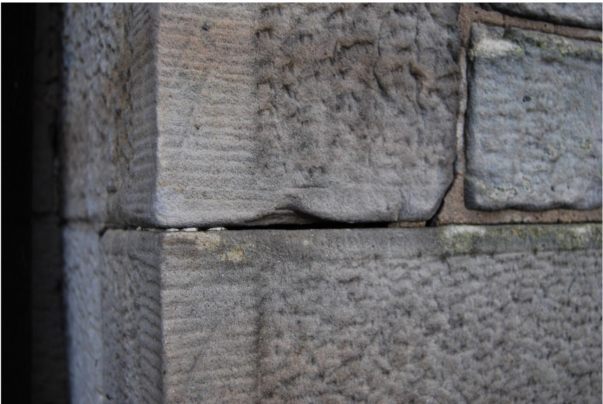
Figure 6: Loss of mortar in masonry joints could be allowing water ingress
