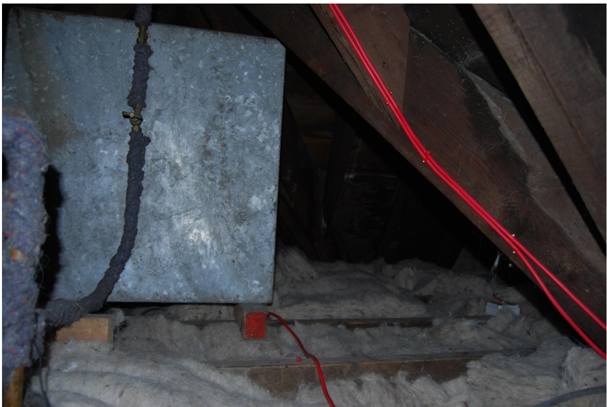
Figure 32: Old water tank in northern attic space which blocks access to far side of attic space.
