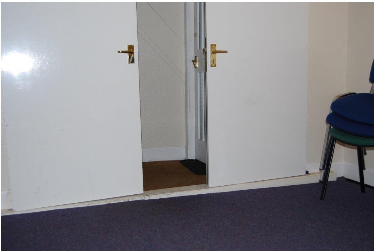
Figure 16: Uneven floors due to movement from settlement.
