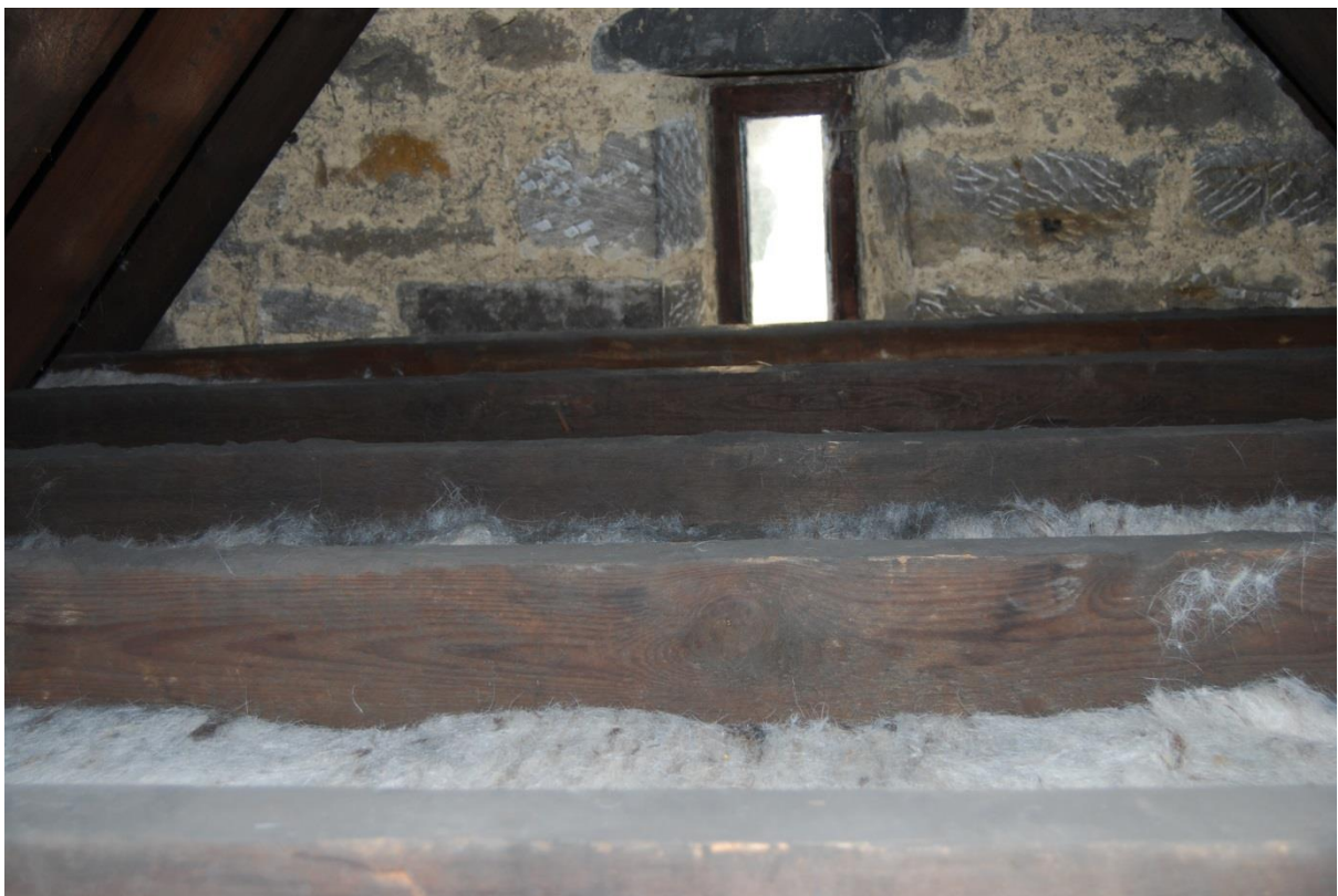
Figure 28: Southern attic space looking south showing small amounts of insulation and no mould.
