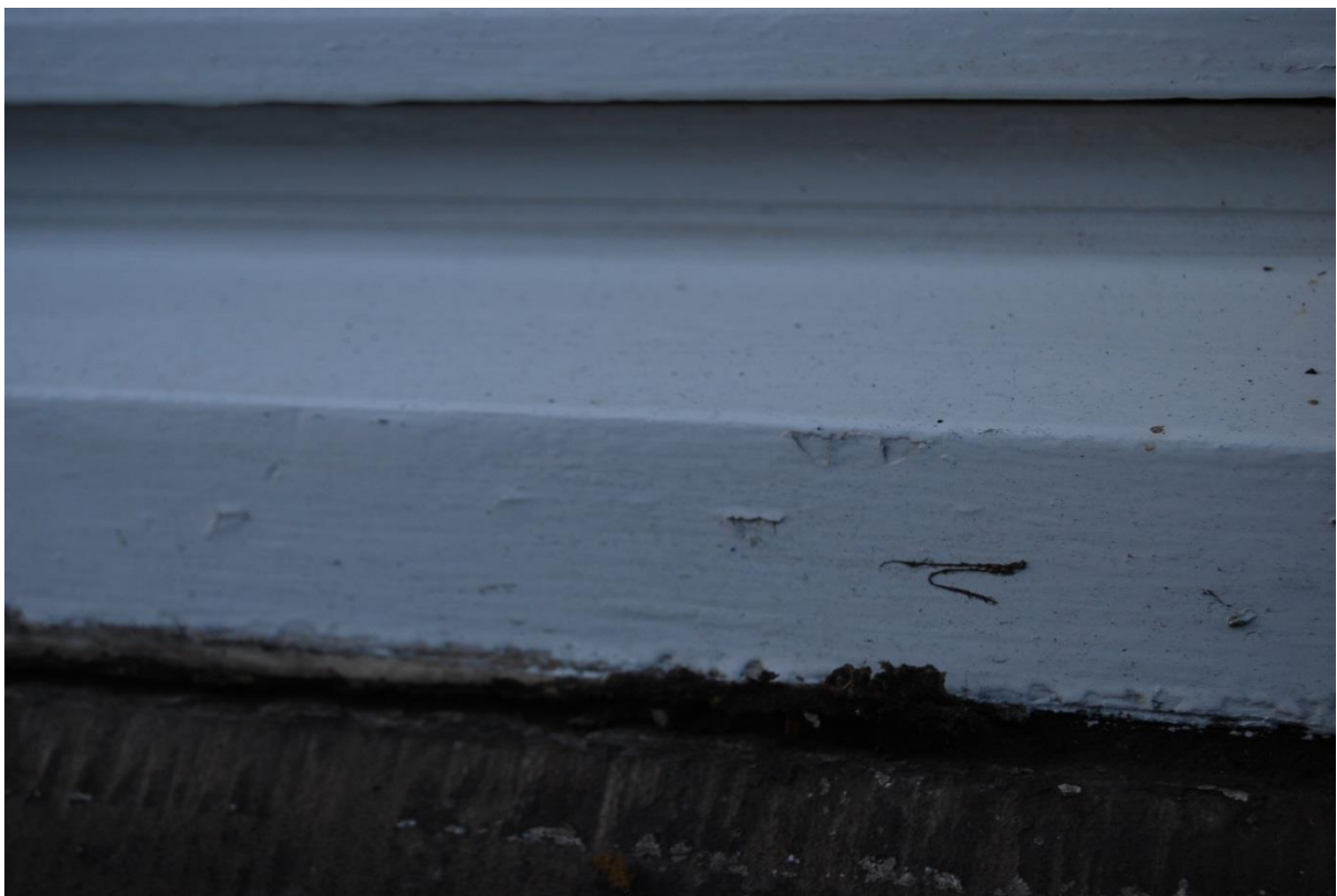
Figure 10: Mastic which has peeled off exposing the mortar joint below.
