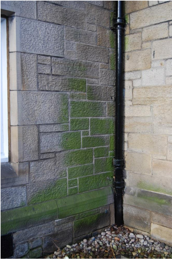
Figure 5: Greening on masonry due to excess moisture
