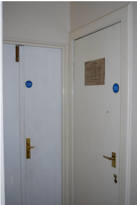
Figure 22: Fire door on boiler cupboard beneath the stairs.
