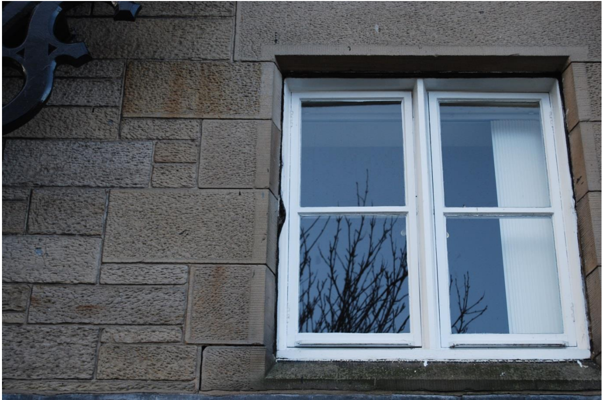
Figure 9: Warped mastic around the window which could be allowing water ingress.
