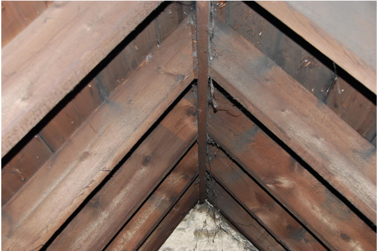
Figure 29: Rafters and ridge beam of southern part of the roof in good condition.
