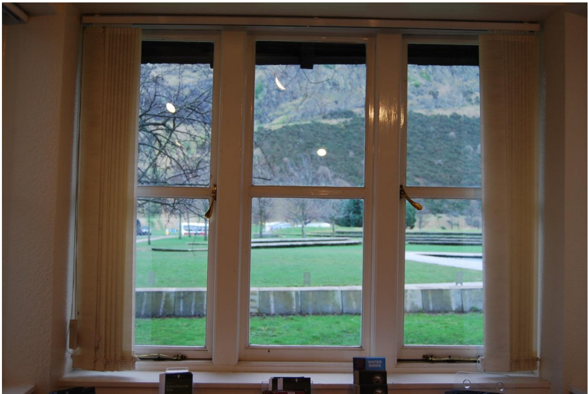
Figure 18: Openable windows on the south elevation with gaps appearing at the bottom due to settlement.
