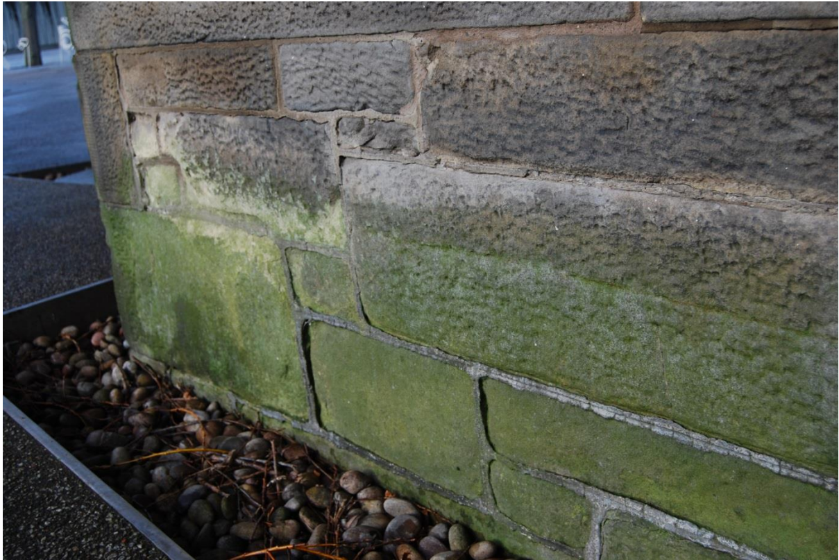
Figure 7: Cement pointing on the lower wall starting to fail.
