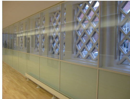
The old façade is preserved by adding floor-to-ceiling glazing on the inside.
