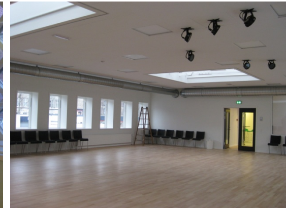
Daylighting and natural ventilation via roof windows.
