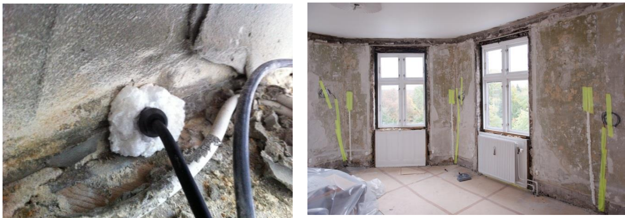
Figure 47: Placements of sensors behind beam-ends (left), drilled and sealed with foam, and in notches in the interior render (right), notches for the wire sealed with foam
