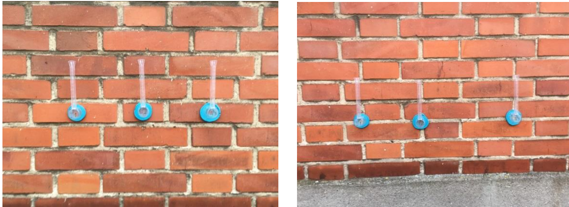
Figure 60: Karsten tube measurements on Bricks (left) and joints (right) for RIBuild case study building in Haderslev (Denmark).
